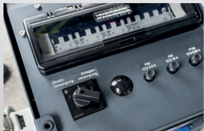
Switch for changing from direct supply to system supply.
